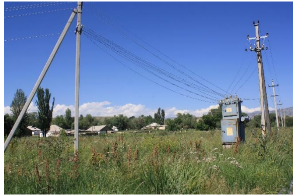
Figure 20: transformer in Jergetal
