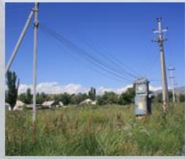
Stack 1: transformer in Jergetal
