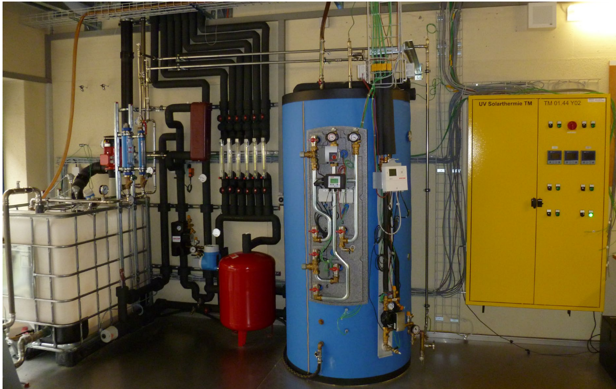
Fig. 5: Solar thermal Laboratory of the Institute of Energy Systems and Fluid Engineering (IEFE). Solar energy storage tank (blue), large reservoir as a reference for short term measurements (white)
