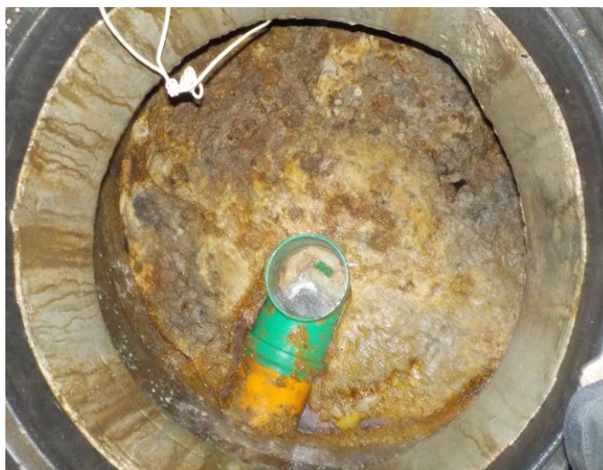
Figure 33: Thick scum layer in settler P1, July 4, 2018
