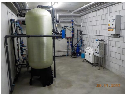
Figure 8: Pressure sand filter (PSF) located in the plant room. Picture: Autark Engineering AG, (2018)
