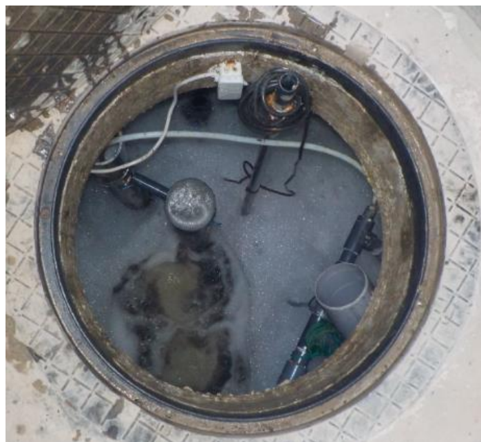
Figure 13: Strong foam formation in the aerobic reactor on Aug. 14, 2018
