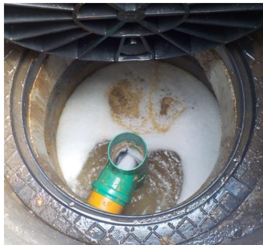
Figure 19: Shock load of washing water in settler P1 reported on Aug. 14, 2018. The shock like entry caused the water to flow over the scum and the water level rose rapidly, covering the entire surface in the settler.
