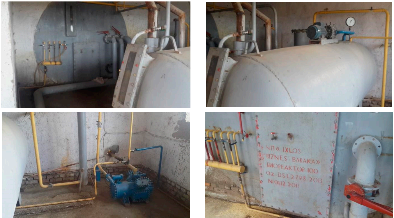
Figure 2. Biogas plant of the Agrofirma.
