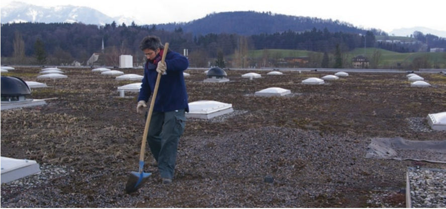
Fig. 2.4 Setup of uneven topography on a green roof. In order to enhance plant and animal (e.g. arthropod) biomass, the environmental conditions of some of the selected roofs were improved by adding a layer 8–16 mm-thick of expanded slate on the pre-existing substrate (30 mm-thick layer of pumice lava and clay) hosting sparse ‘moss and Sedum spp.’ vegetation. (Photo credit: Nathalie Baumann 2009)
