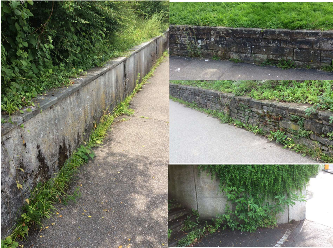
Figure 49 Left wall ID 22, right top down: wall ID 33, 23 and 1 (pictures: S. Caregnato)
