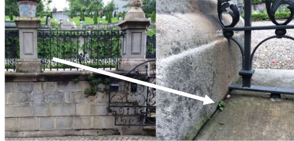
Figure 17 Retainment wall with balustrade on the wall top of wall ID 8 (photo: S. Caregnato).
