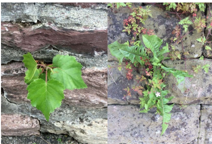
Figure 19 Left example of strong roughness, right example of weak roughness on vertical wall surfaces (picture: S. Caregnato).
