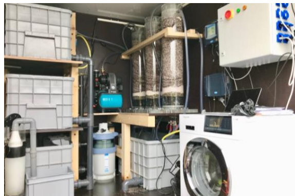
Figure 2: Interior of the LaundReCycle prototype including washing machine and installations for the water treatment
