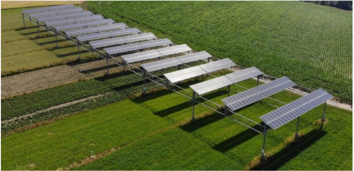
Figure 2: System example for "open arable crop" management status. Agri-PV trial system (APV Resola) with non-tracking modules in Heggelbach (Germany). The modules are installed at a height of 5.5 m and the distance between the supports in the longitudinal direction is 19 m (Hofgemeinschaft Heggelbach, n.d.).
